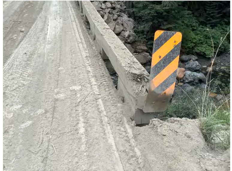
Impact of rail, downstream right. Rail still solid and not loose
